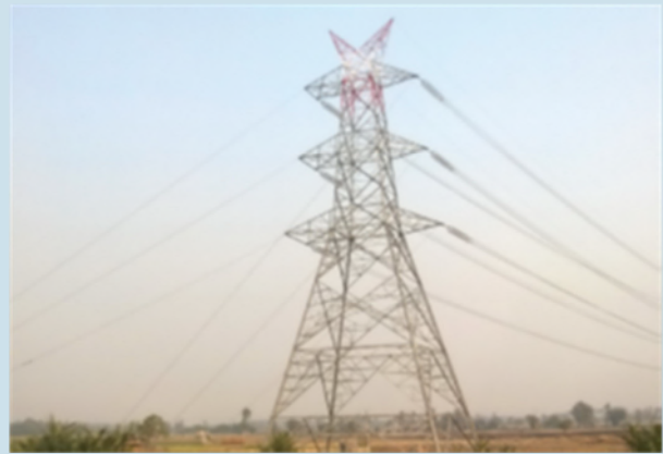
Power lines in India. In order to prevent bottlenecks in the grid, many thousands of kilometres are to follow Source: KfW Group, photographer: Walter Klotz
