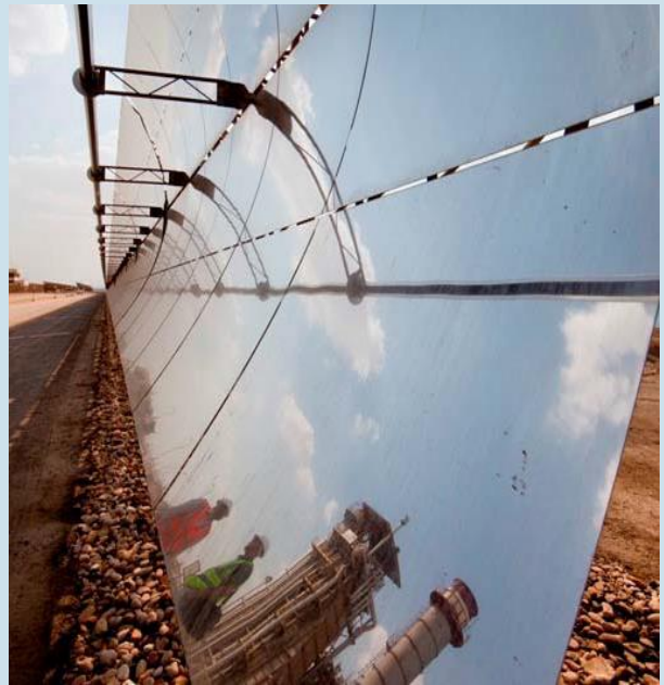
Parabolic mirrors at the solar power plant. Source: KfW photo archive, photographer: photothek.net
