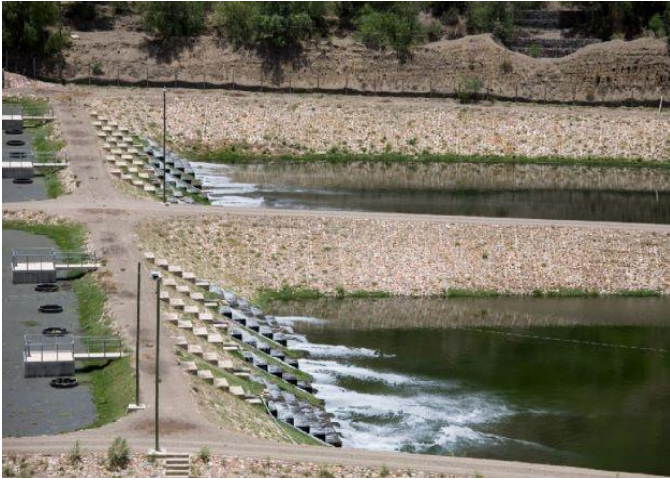
Wastewater treatment in a wastewater treatment plant. Source: KfW photo archive / Bernhard Schurian
