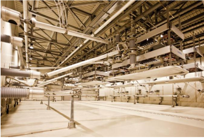
Energy alliance: Substation in Georgia. Source: KfW photo archive / Rendel Freude
