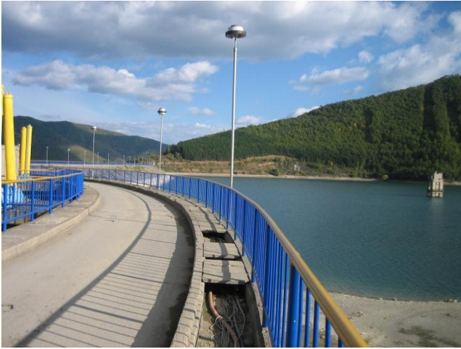
Gazivoda Lake is to be exploited as an additional source of drinking water for Pristina. Source: KfW/Dr Karl-Dankwart Kummer
