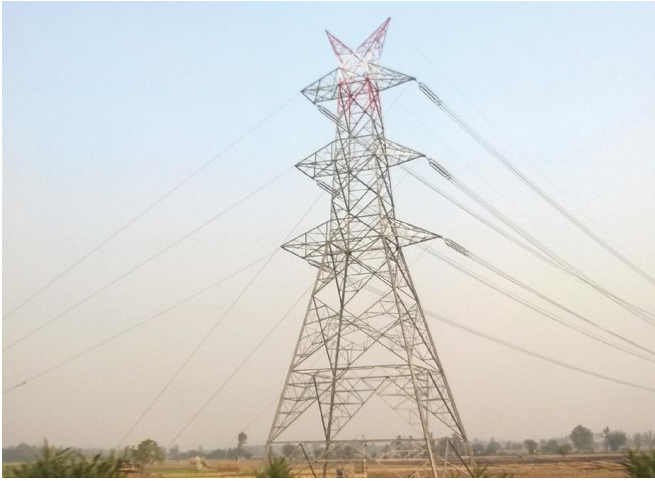
Power lines in India. To prevent bottlenecks in the grid, many more thousands of kilometres are still to follow. Photo: Walter Klotz
