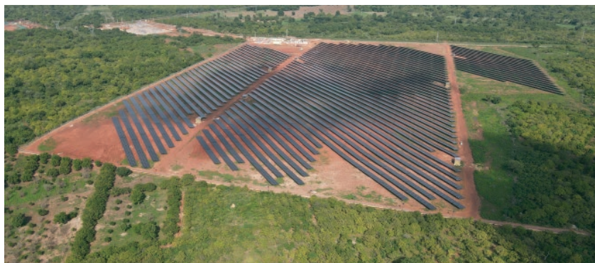
The solar plant in Boundiali is considered a lighthouse project in West Africa and promotes the ambitious climate goals of Côte d'Ivoire.
