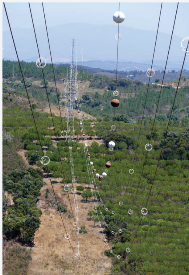
Multiple bird flight diverters installed on a transmission line. Algarve region, Portugal. Photo: Alvaro Camiña
