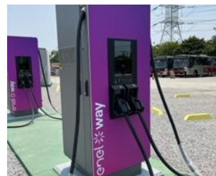
Charging station in São Paulo, Brazil.
