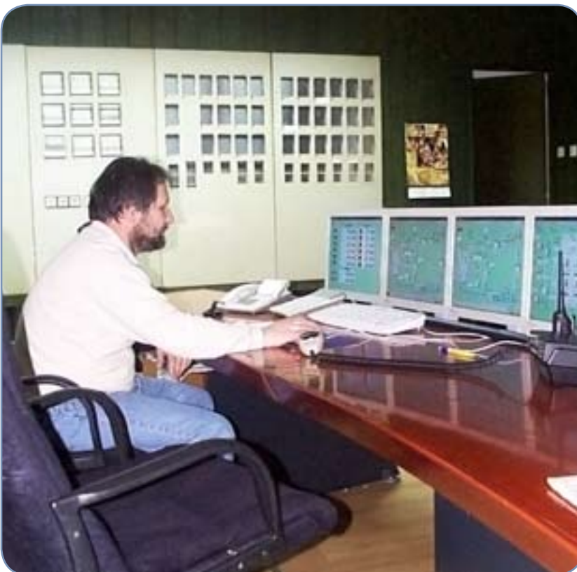
The switch and control centre for the district heating network in Belgrade.
