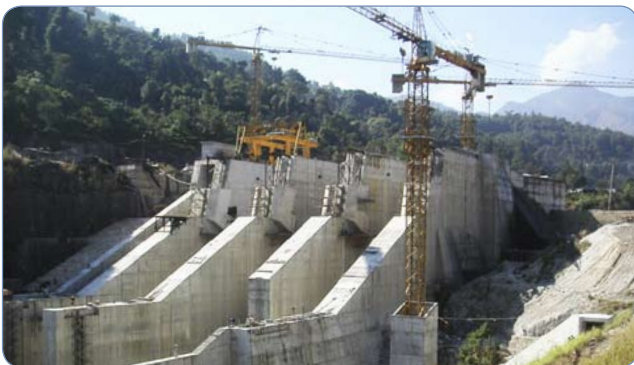
The upper section of the Middle Marsyangdi hydropower station.
