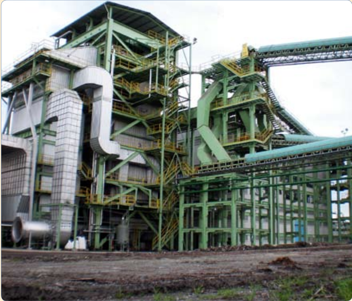
Bagasse power plants produce steam and electricity from sugar cane waste.
