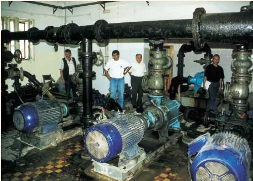
Fast reconstruction in Kosovo through FC: repairing the drinking water supply in Prizren.
