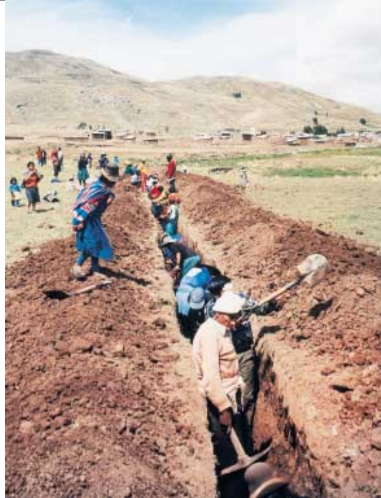
Helping people to help themselves in the water sector.
