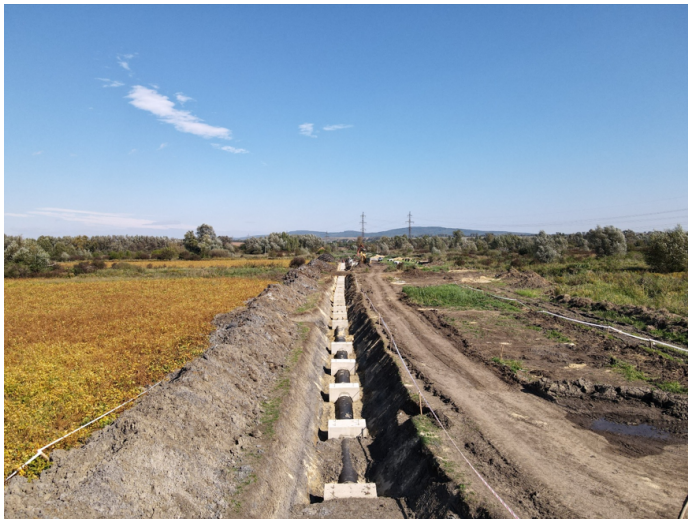
A water pipe is being rehabilitated in Chernivtsi. Image Source: Hennadii Dudko, Strategic Development Department Chernivtsivodokanal
