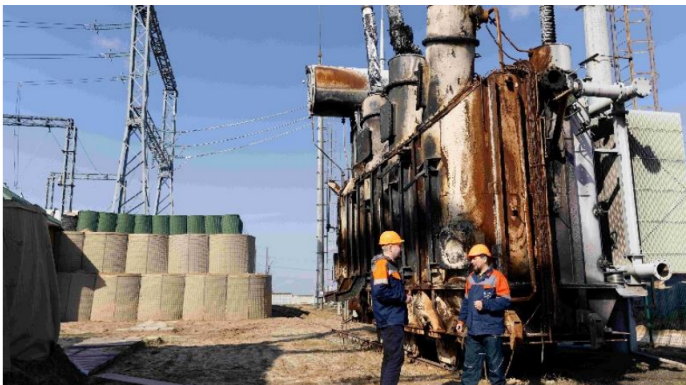
Ukrenergo employees stand in front of a transformer hit by a drone in central Ukraine. Image source: KfW Photo Archive / Jonas Wresch
