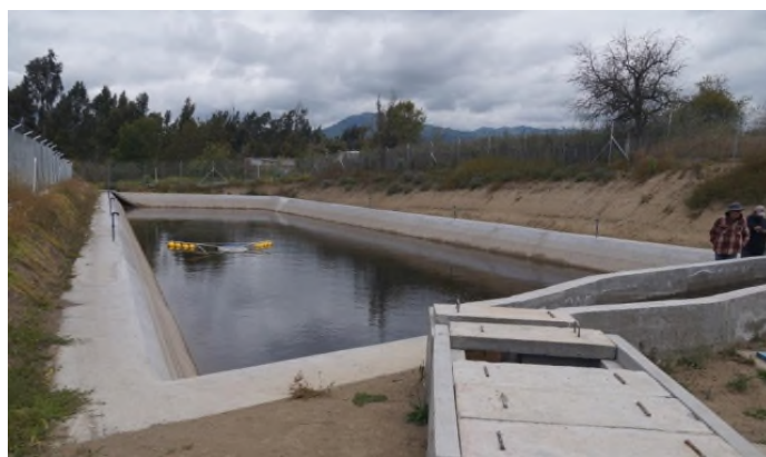
Main storage basin. Source: KfW / Michael Heiland
